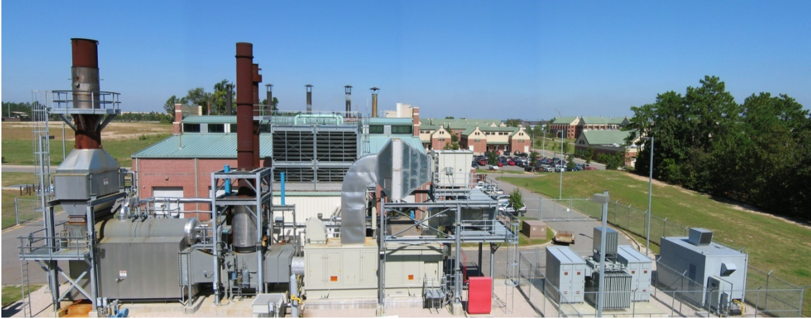
Figure 2: Ft. Bragg CHP Installation
